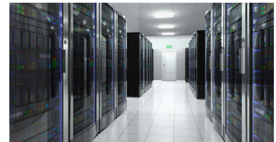
The large additional electrical consumption metered in Tower Hamlets is likely to be from server rooms and trading floors in Canary Wharf. These are not reported on building Display Energy Certificates (DECs). Image courtesy Green Cooling
